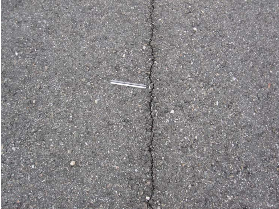
R1836JK-10. Longitudinal and Transverse Cracking (Sample Unit #45).
