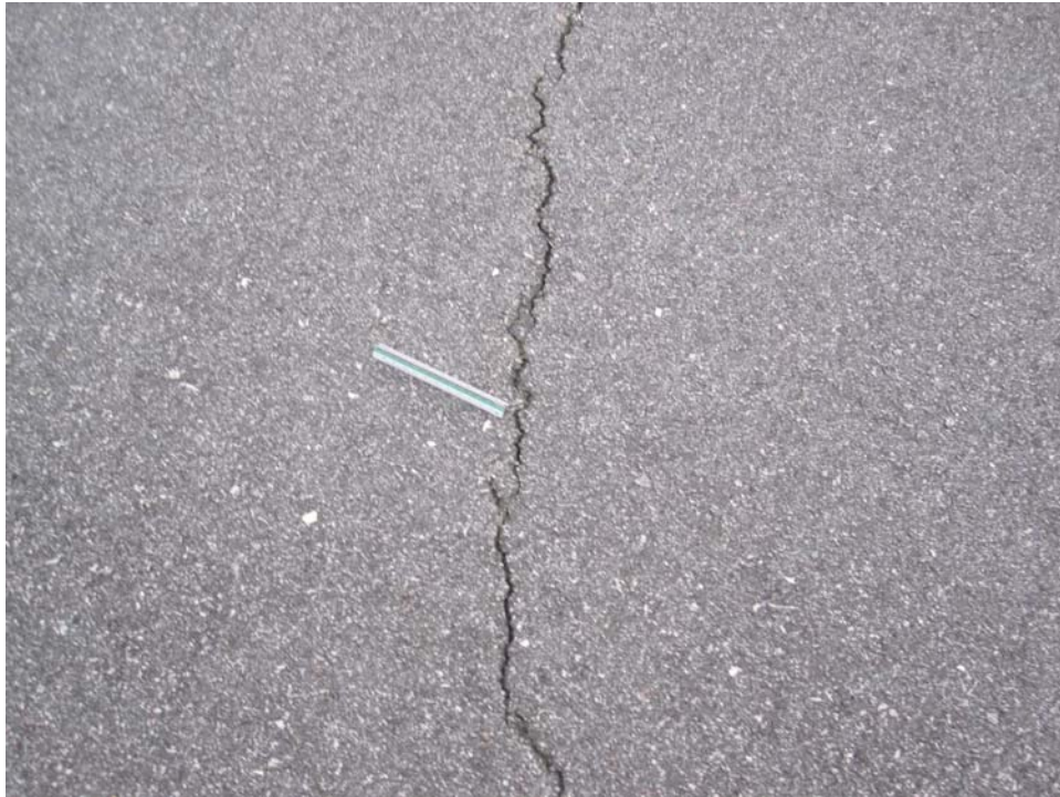
A01JK-10. Longitudinal and Transverse Cracking (Sample Unit #02).
