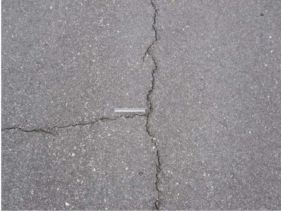
TAJK-10. Longitudinal and Transverse Cracking (Sample Unit #03).
