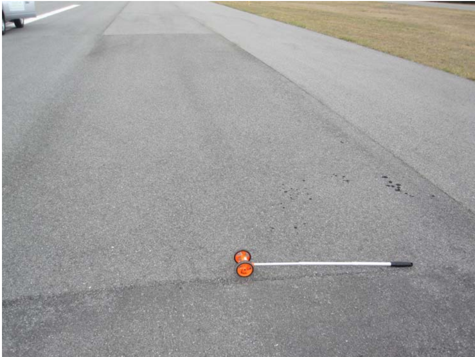
R1836JK-10. Patching (Additional Sample Unit #31).
